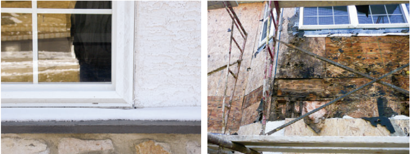
Figure 1. When the author investigated this home's leaky windows, he found that the stucco was tight against the window frames — an indication that no casing bead had been installed (left). When the stucco was removed, extensive rot was discovered in both sheathing and framing (right).
